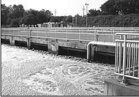
Aeration tank at Columbia Blvd Wastewater Treatment Plant (Image from City of Portland Website)
